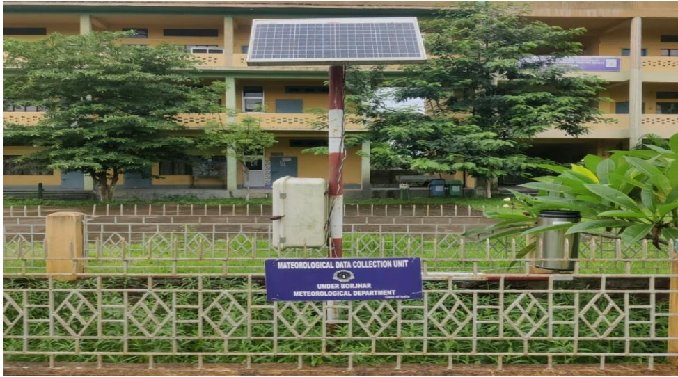
METERIOLOGICAL DATA COLLECTION UNIT GOVT OF INDIA
